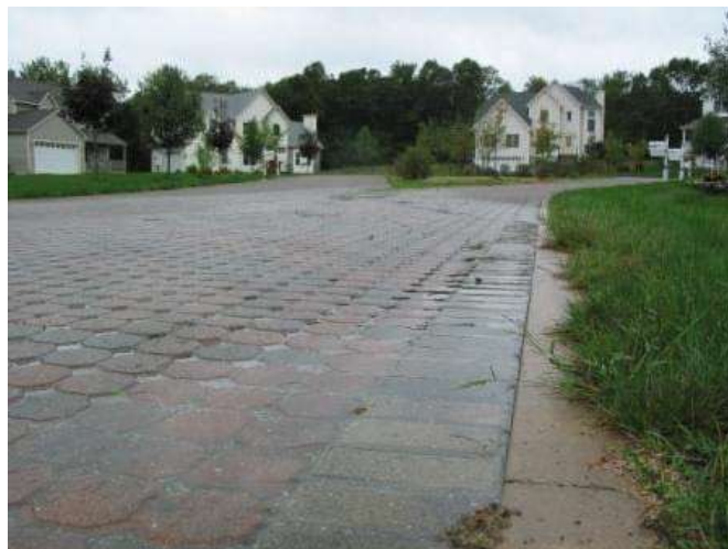
Exhibit 10-8. Jordan Cove Permeable Pavement (UConn, 2007)
